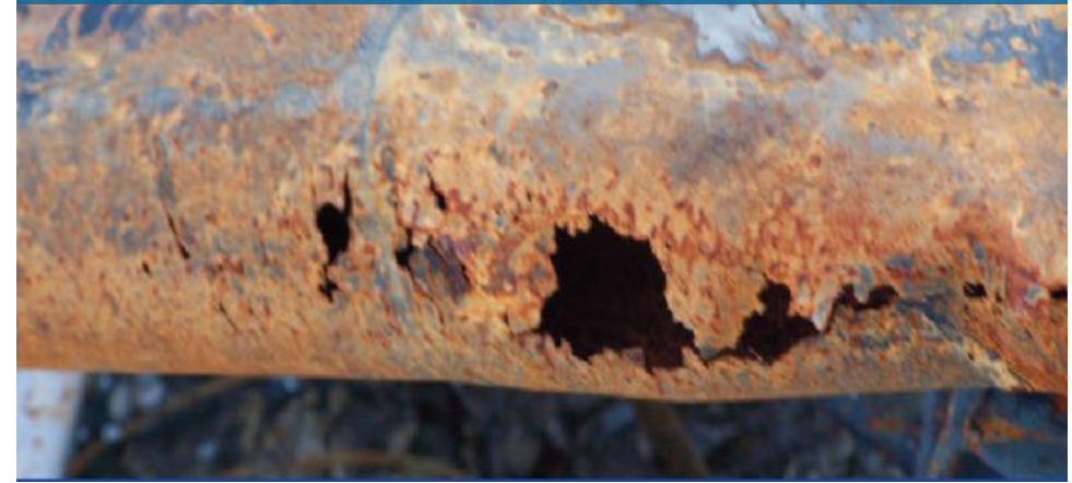
CUI on pipe causing perforation
