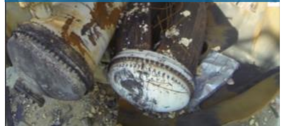
CUI-induced heat exchanger in olefins plant 3
