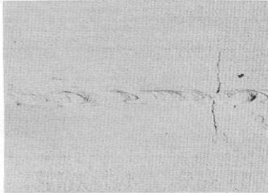
Fig. 6 Stress corrosion cracking observed on a welded vessel used as a storage for industrial grade methanol.
