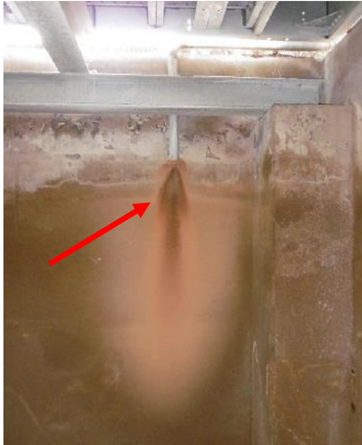
WELL WATER INJECTION
