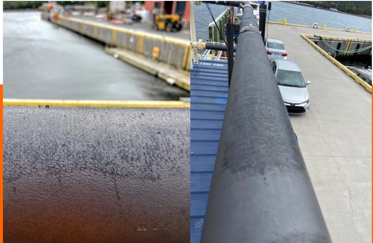
Tarpaulin Residue welded to CIDS coating
