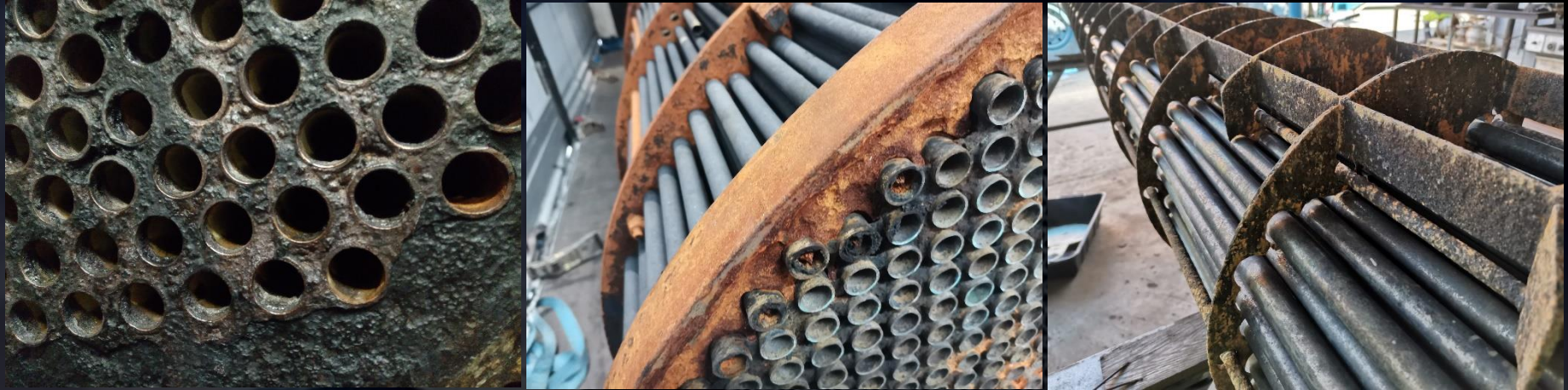
Corrosion due to interaction between metals with different potentials
