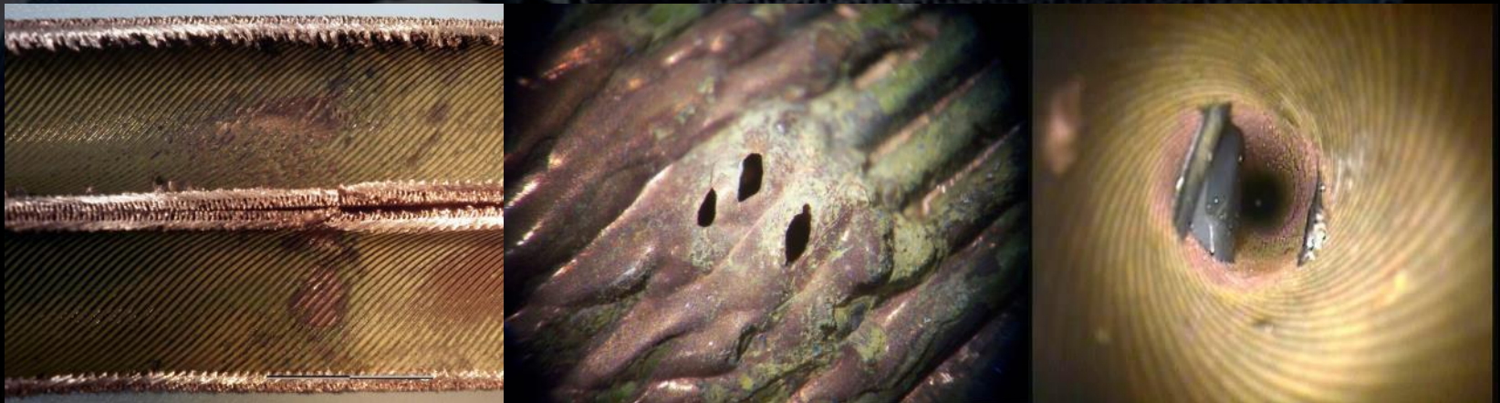
Over velocity erosion in copper tube due to presence of foreign materials
