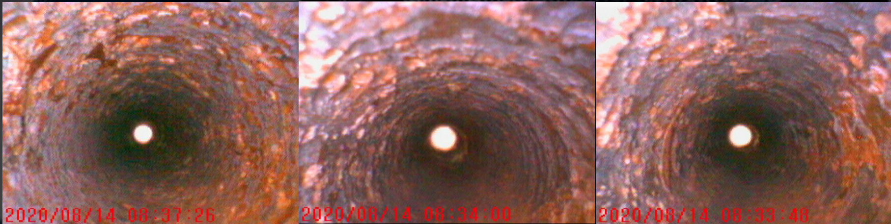
Erosion in Cu-Ni tubes due to presence of sand
