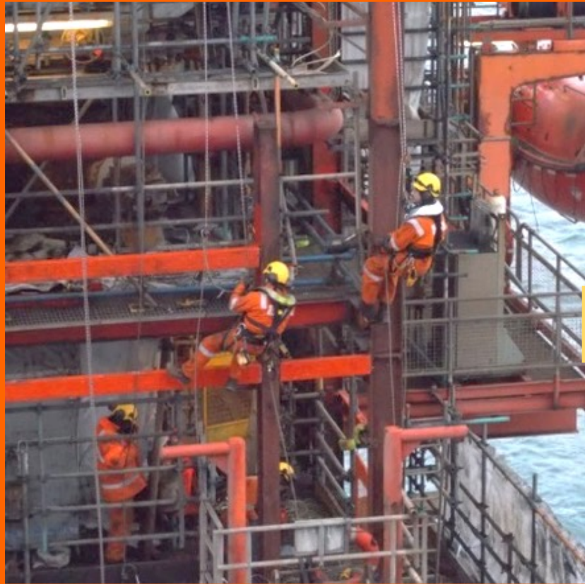
Manual Hunting – Visual / NDE Inspection
