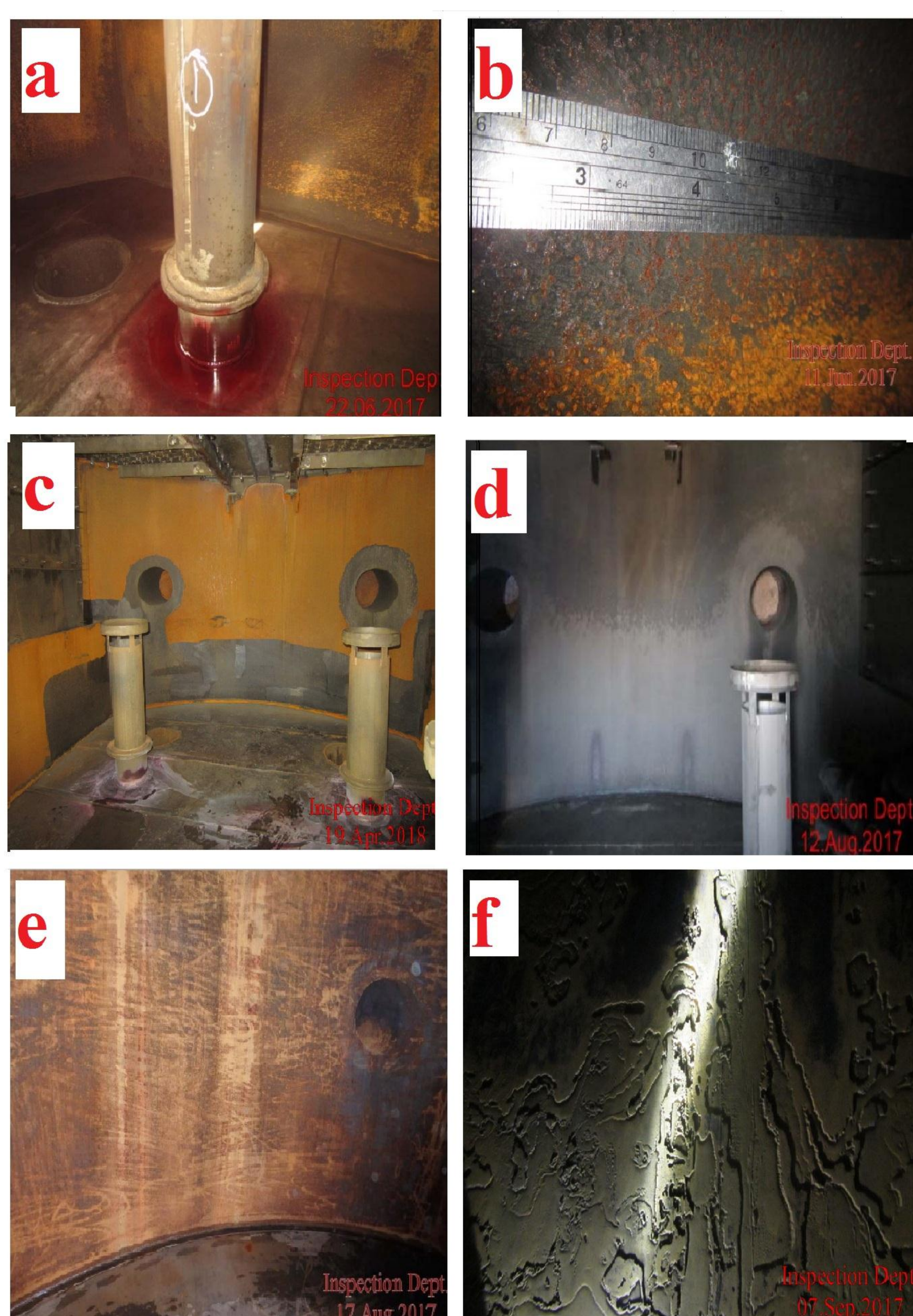
Figure 1: Comparison of corrosion extent in different amine treating units: a) Chimney tray area of GTU1, b) Chimney tray area of GTU 3, C) Chimney tray area of GTU4, d) Chimney tray area of GTU 5, e) Chimney tray area of GTU 6, f) Chimney tray area of SRU
