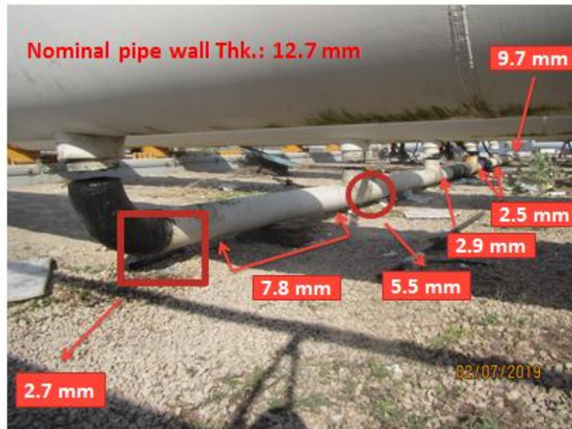
Fig 1: Results of UT measurements on 10 inch equalizer pipe in slug catcher indicated Severe metal loss in this pipe
