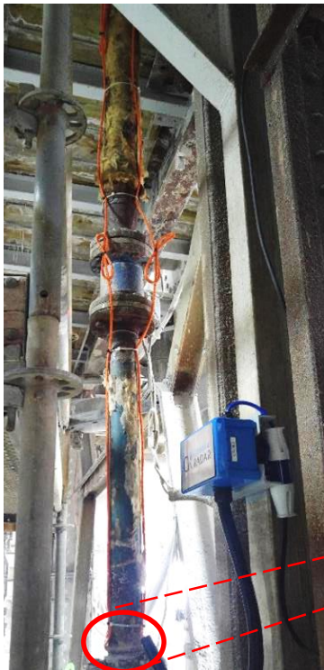
CRL002 – Vertical Pipeline
