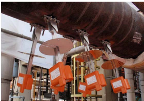
Six sensors installed in close proximity to detect Napthenic Acid attack in refinery
