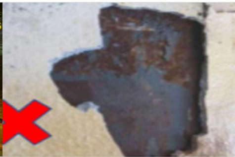
Corrosion under HC PFP
