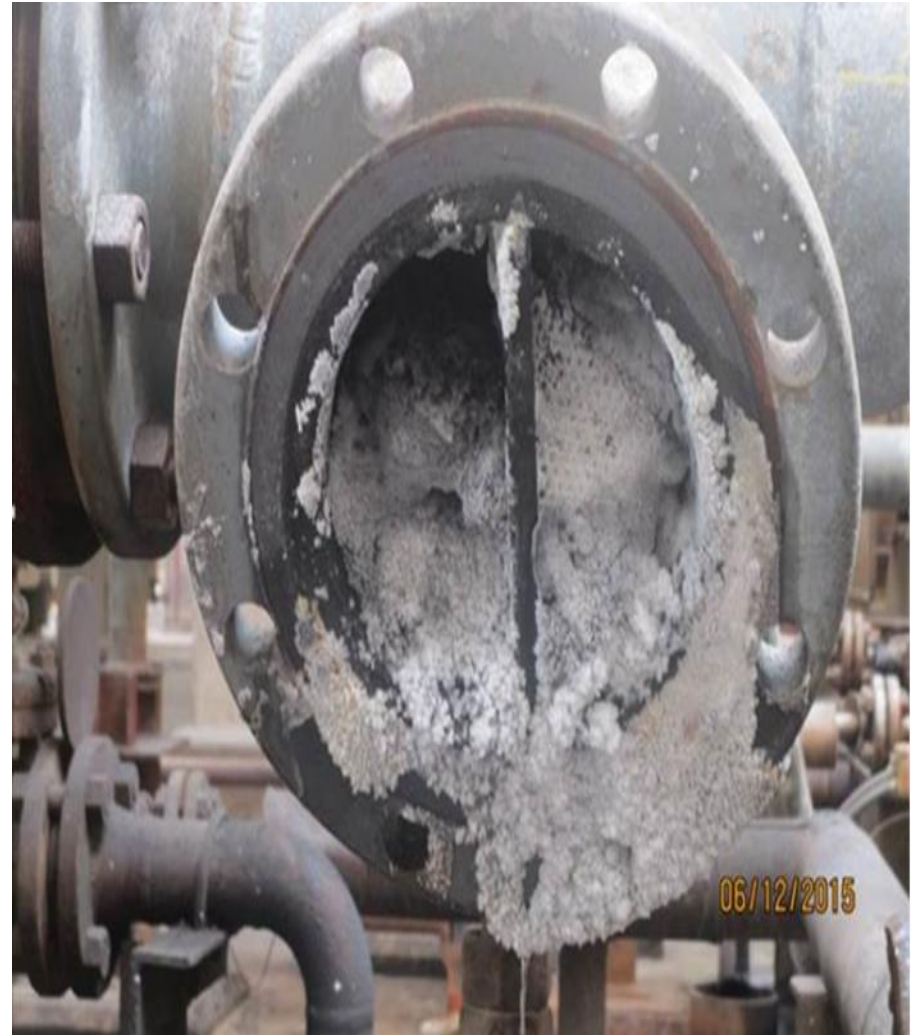
Figure 1: NH 4 Cl accumulation in heavy gasoline pump strainer
