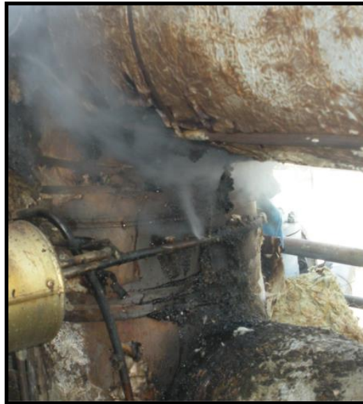
Steam leakage BPA system
