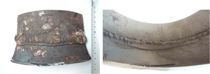
Outside : Crack follows Heat Affected Zone
