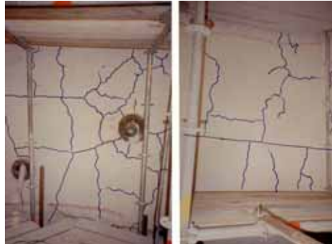
Normal crack pattern in gunnited medium weight concrete
