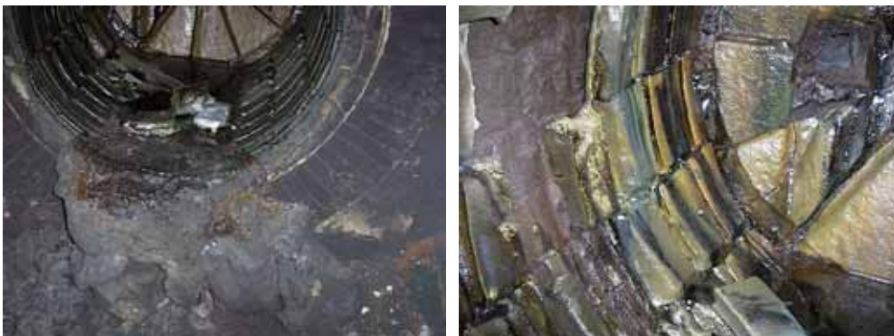
Attack of burner lining by fuel ash
