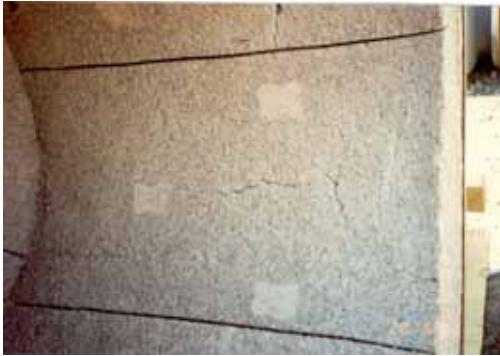
Excessive shrinkage in cold joint increased risk for hot spots
