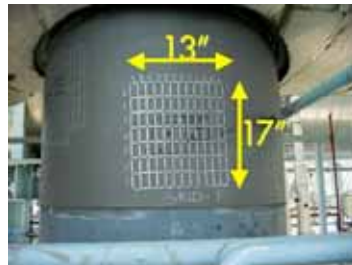
Area with increased corrosion
