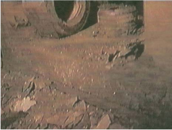
Internals of the reactor covered with sulphide scale
