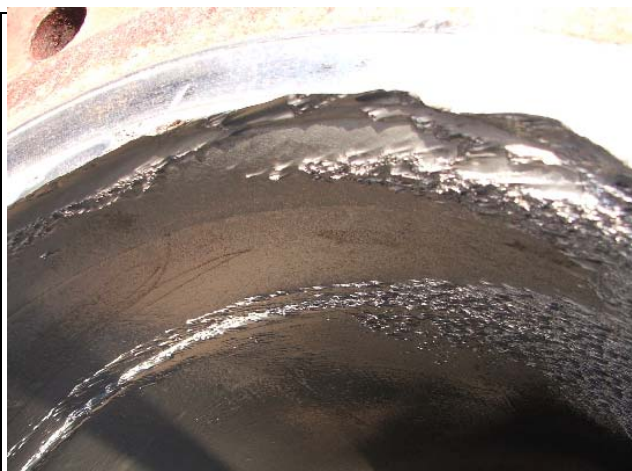
Erosion on the inside surface of a tube header. Dust in the header was composed of graphite, iron, \text{Cr}_7\text{C}_3 carbide, and traces of catalyst material
