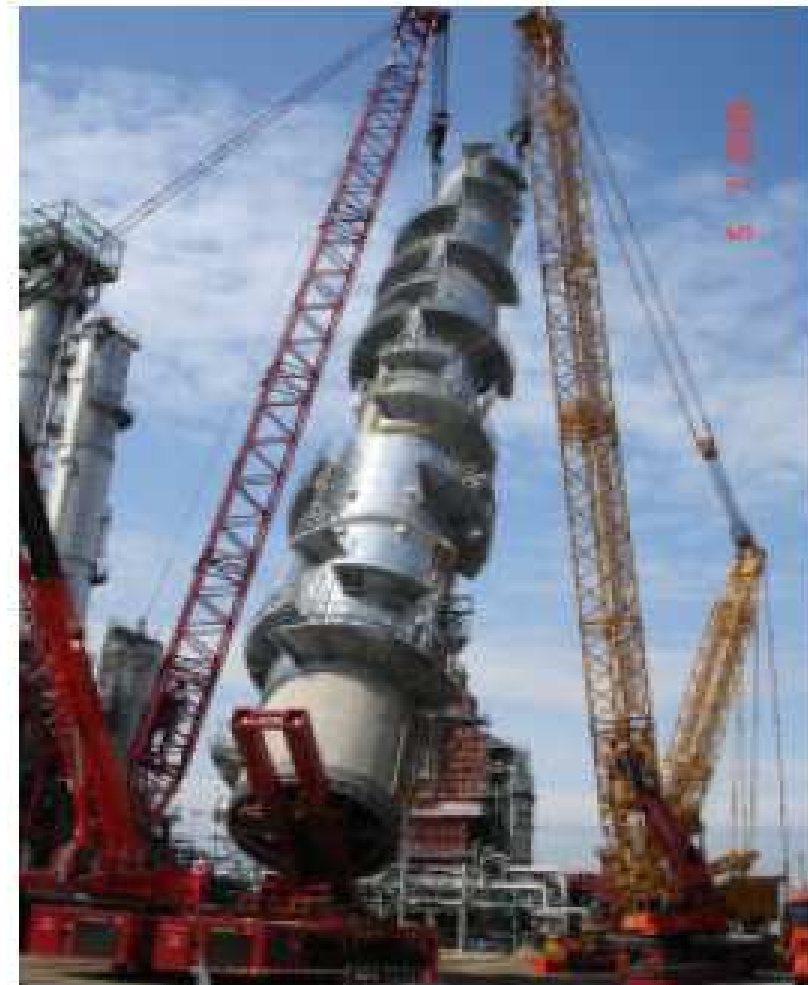
60m high by 5m OD tower - TSA coated
