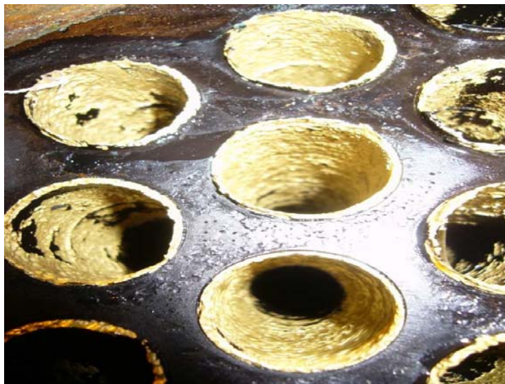
Tube end erosion by high velocity sea water
