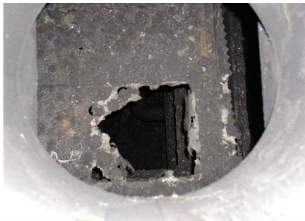
View of a less heavily damaged tray
