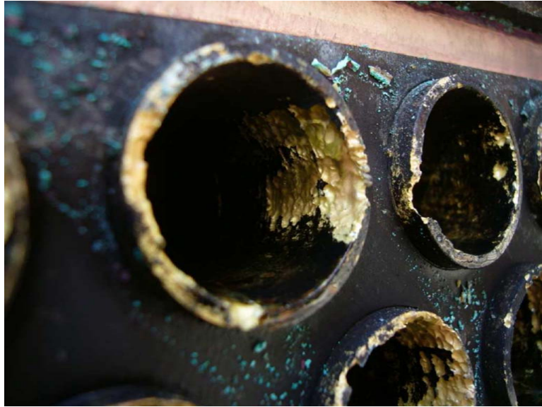
Tube end erosion by high velocity sea water
